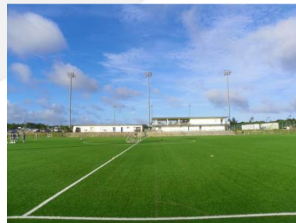
The pitch was installed with regard to Guam’s history of typhoons and heavy rains.
